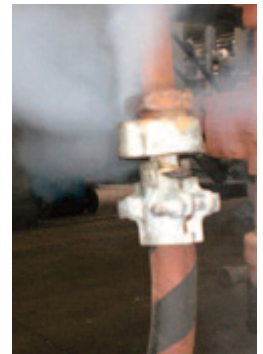
Leaking hoses are dangerous and costly
