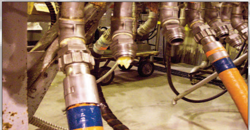
This plant replaced all the cam and groove outlets with Chemjoint outlets due to constant leaks caused by viscous material.
